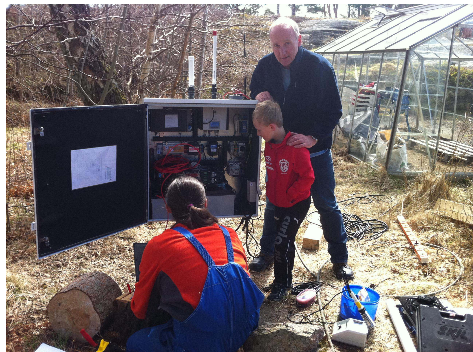
Koljöefjord shore station with GPRS data transmission antenna.
